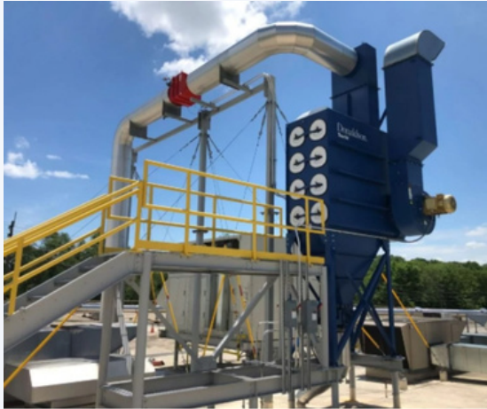
Rooftop-mounted cartridge collector with elevated ductwork run
