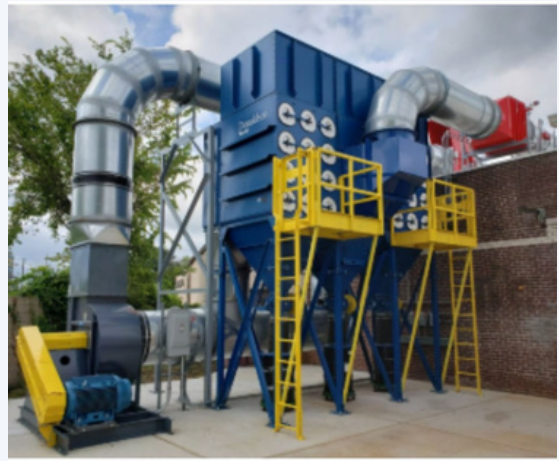
Ground-mounted unit with rotary airlock discharge and access platforms
